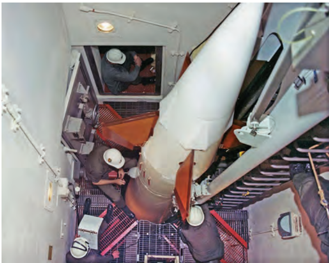
Historic photo of Spartan missile in its silo during installation. Provided by Clint Esciklsen
